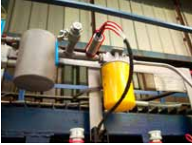
The TRANSEC Units are available with moisture and temperature monitoring in both inlet and outlet oil pipes. The reliable and stable measurement provided by the Vaisala MMT162 is not just a means to monitor moisture in oil, but also a measure for the performance of the moisture management system.
