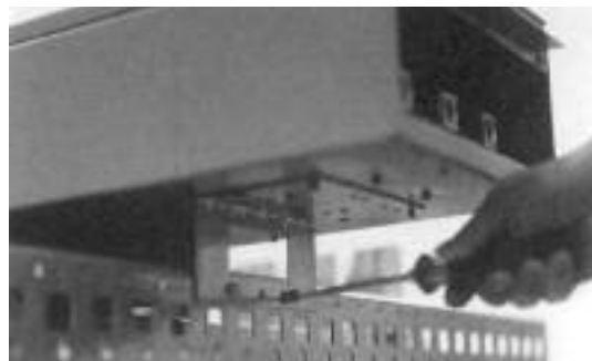
Fusible Switch Module Mounted on Interior
