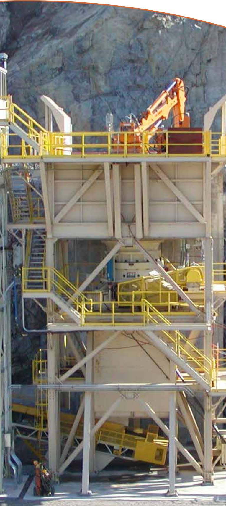
Stationary primary gyratory station
