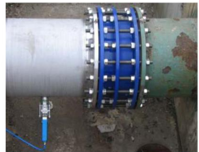
Simple pipe sensor mounting.
