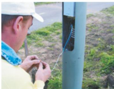
NivuChannel power supply using the street lighting
