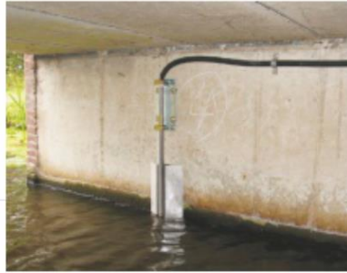
Installed rod sensor with accessories
