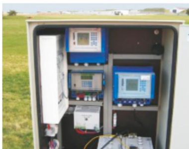
Clearly installed in a switching cabinet
