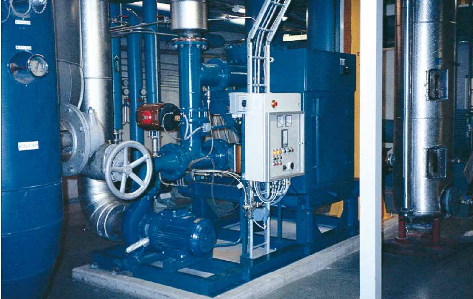
SALA-HGMF® for control of magnetite concentration in a district heat flow of 10.000 m 3 /h.
